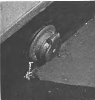
Outlet for vacuum cleaner system
