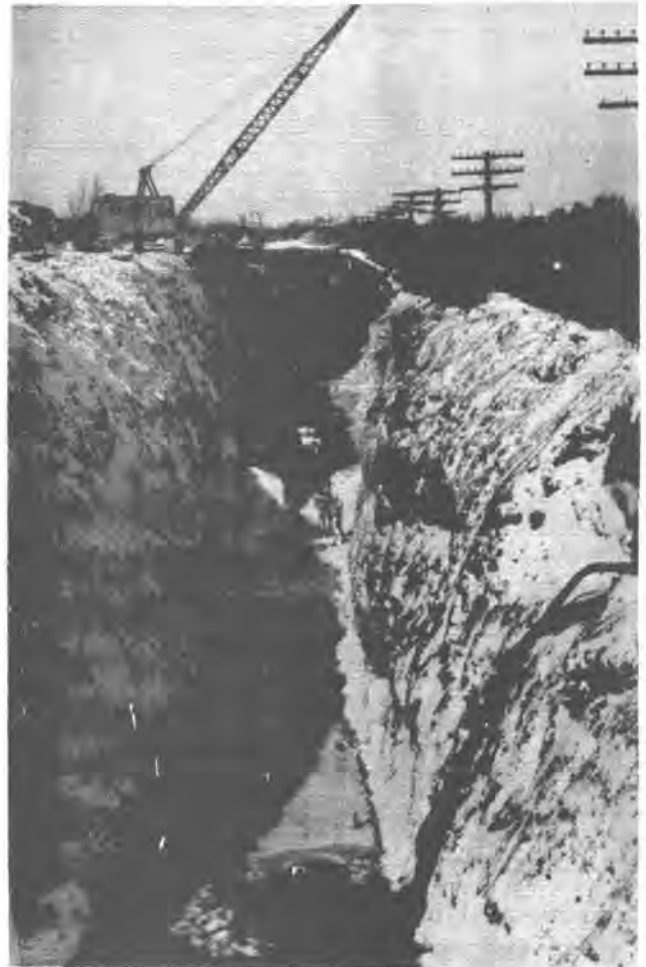
Lexington Avenue sewer, here shown in process of building will soon be an underground river
